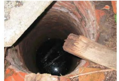
OPEN WELL CASING. Improperly abandoned wells can transmit contaminants from the surface into groundwater and can also be a safety hazard to people and animals. This open well casing is an example of an abandoned well that has not been properly filled and sealed. Source: Groundwater Resources Association of California: http://cart.grac.org/Abandoned-Wells-1?search=Abandoned%20Wells .
