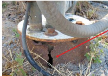
1 CRACKED WELL CASING. A cracked well casing may allow surface water and contaminants into the well. Consult a water quality professional, such as a licensed well driller, to repair or replace the cracked casing. Source: CA State Water Resources Control Board, https://www.waterboards.ca.gov/gama/docs/wellowner_guide.pdf .
