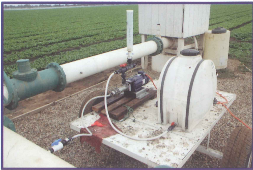
Figure 2: Trailer outfitted for injecting liquid PAM into the main line of an irrigation system using an auger metering pump.
